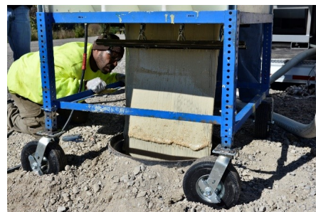
Figure 3. Grout added to funnel and fed into liner grooves which prevents grout from "scraping off" during insertion.
